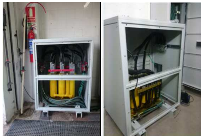
Voltage stabilizers installed at Plaza Mayor
